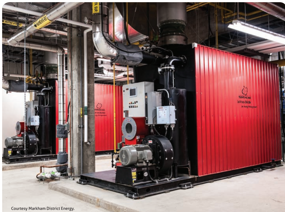
Courtesy Markham District Energy.
